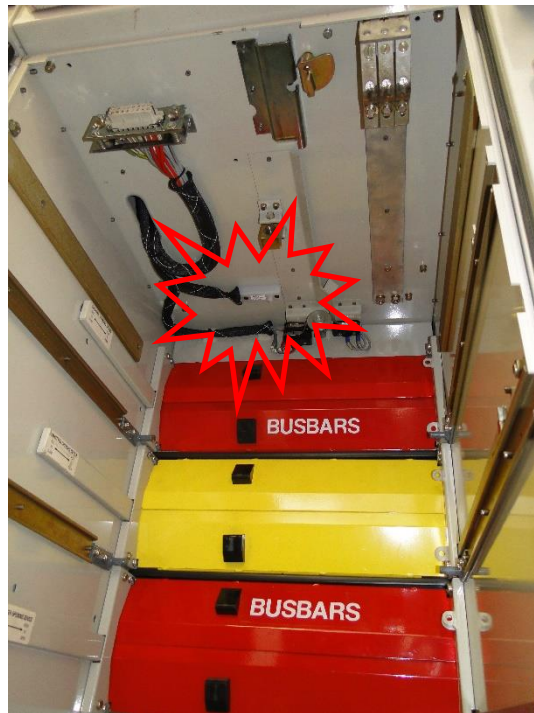
Sensor placement inside the CB racking chamber
