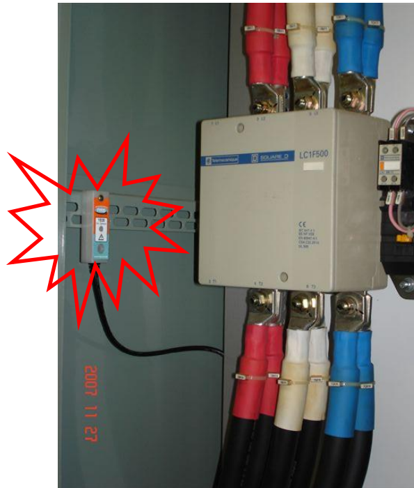
Sensor placement near a Low Voltage Contactor for a Variable Speed Drive
