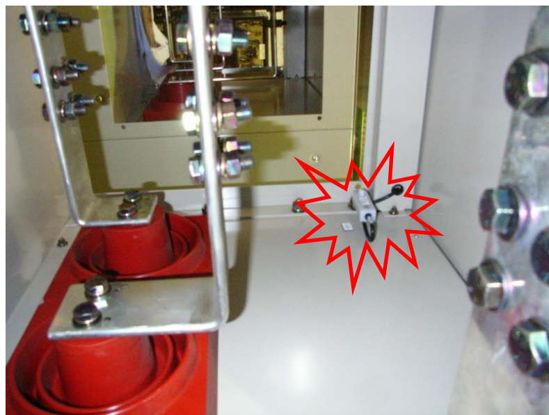
Sensor placement inside the busbar chamber
