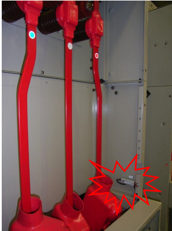
Sensor placement inside the cable termination chamber
