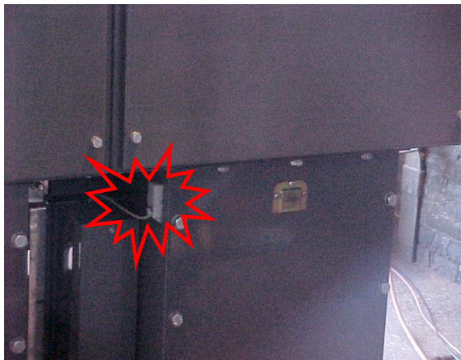
Sensor placement for a Switchgear cable termination chamber (External through Hole Detector)
